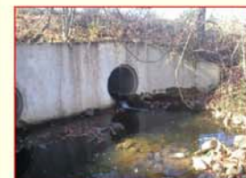
4 End Wall discharges to waters of the Commonwealth of Pennsylvania.
